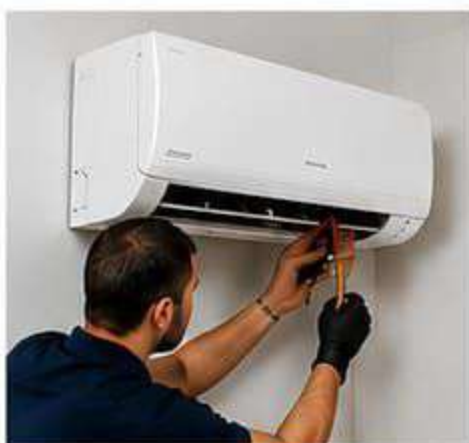
AC INSTALLATION (ALL BRANDS)
