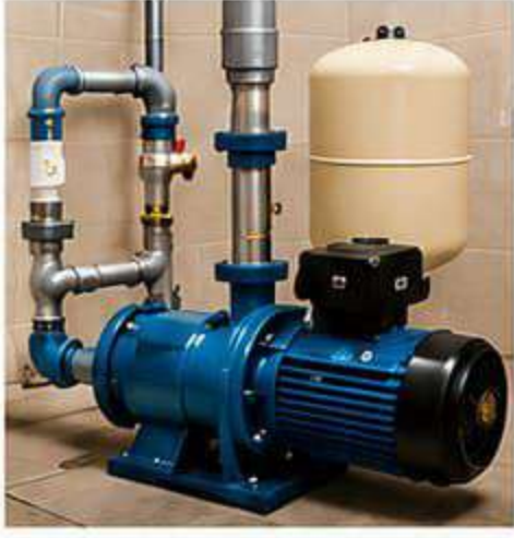
WATER PUMP INSTALLATION
