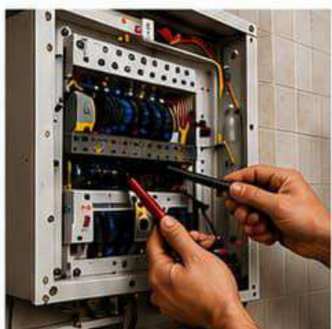
ELECTRICAL REPAIR & MAINTENANCE
