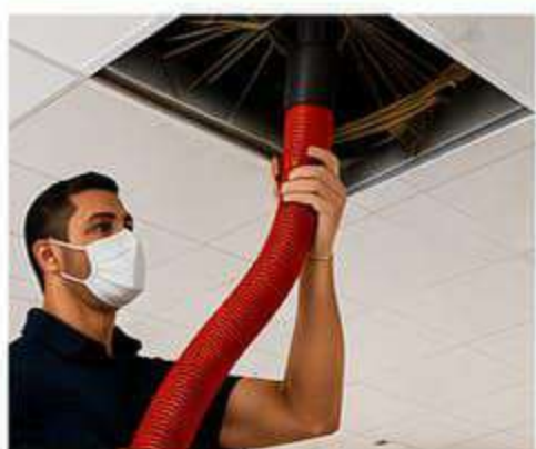
AC DUCT CLEANING
